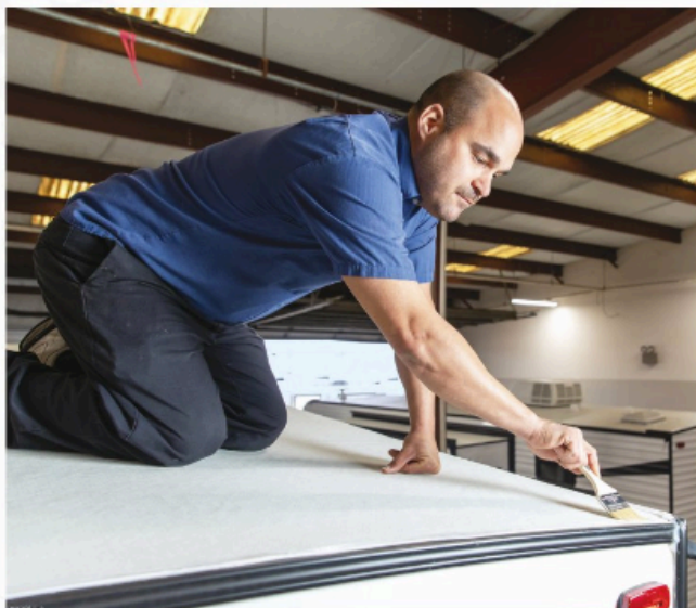
Service Technician Yorniel "Gordo" Suarez applies roof sealant to an RV. Suarez, who has worked at the dealership for seven years, was born in Cuba but became a U.S. citizen in 2017.
